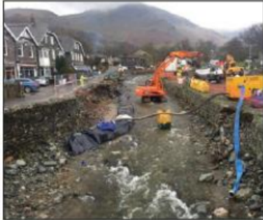
Glenridding village river channel blocked by boulders
